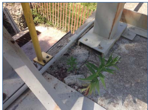
Figure 3: Localized Concrete Spall
