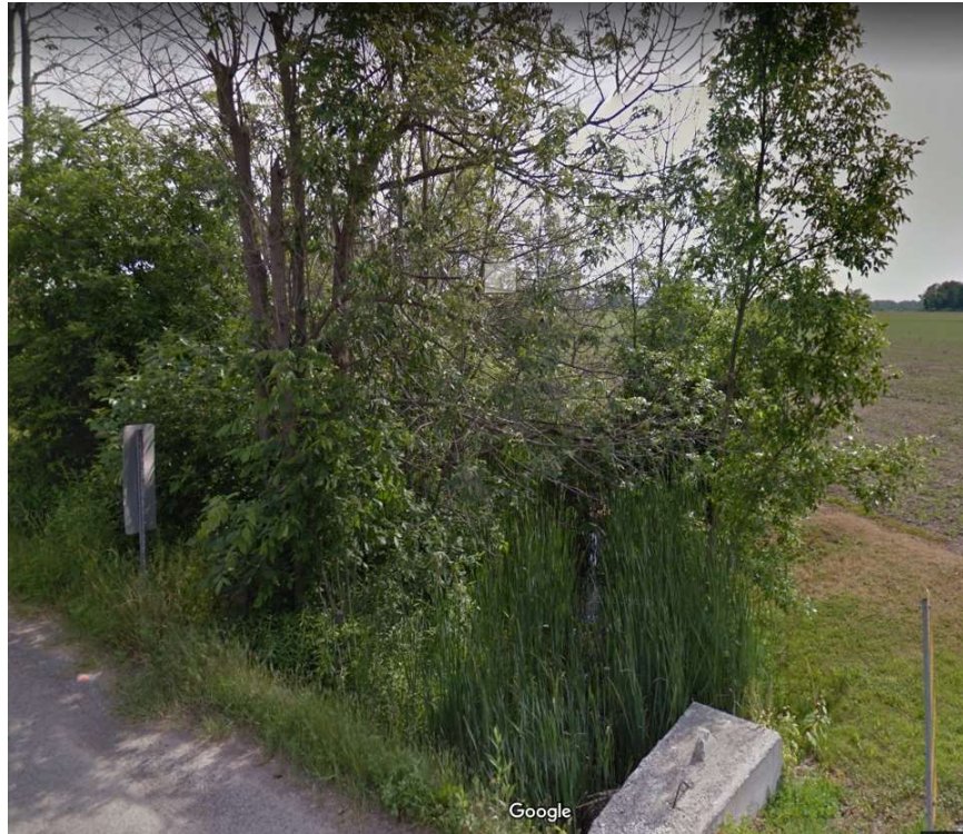
Figure 7 Obstructed drain; Wignell @ East side of Weaver Road
