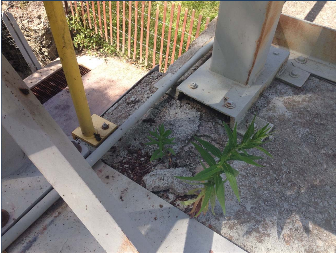
Figure 3: Localized Concrete Spall
