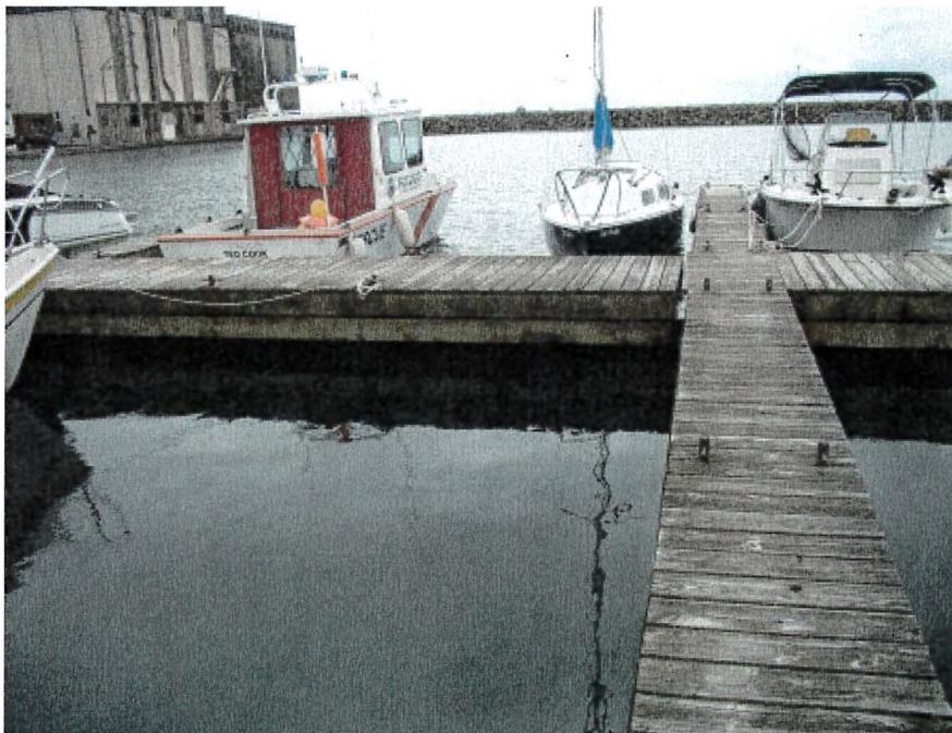
Photograph 64: East Main – Dock 6. Moderate Wear and Rot on Deck Timbers
