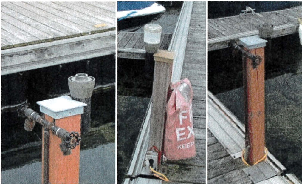
Photograph 82: West Main – Dock A. 3 Light Poles with Lights Missing
