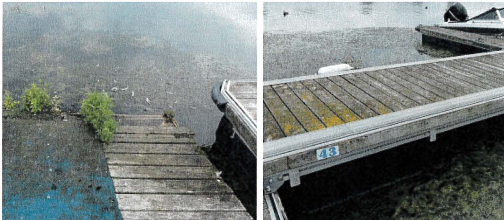
Photograph 156: West Main – Dock J. Moderate Moss Build-up and Lichen on Deck Timbers
