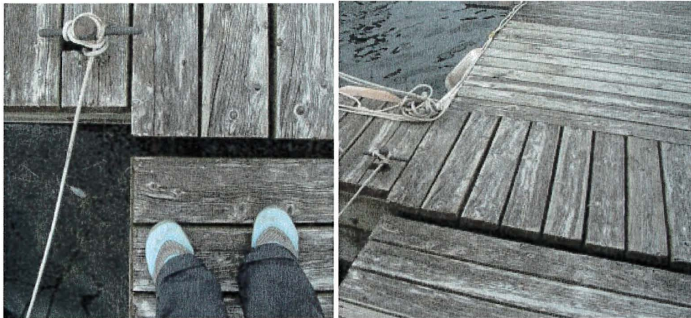
Photograph 65: East Main – Dock 6. Differential Settlement (1 inch) and Gap (2 inches) at Dock-Finger Joint
