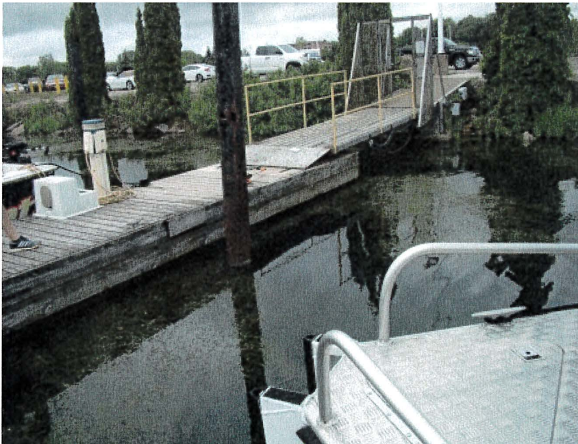
Photograph 22: Dock 2 – Access Gangway. Loss of Buoyancy. Signs of swamping/rotting
