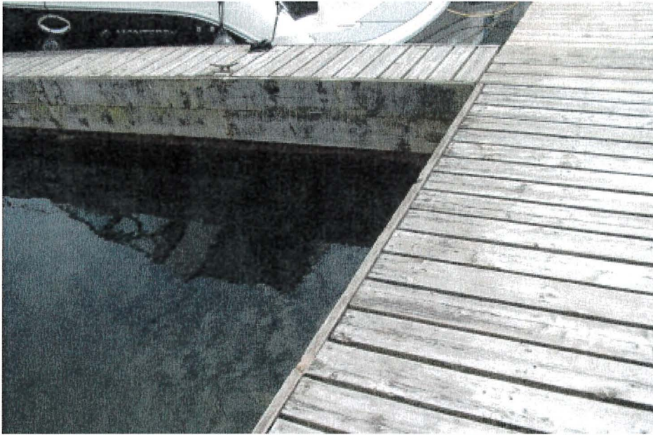
Photograph 15: Dock 1 – Access to Finger 23/25. Timber Discoloration and Moss Build-up
