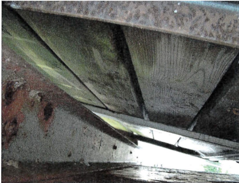
Photograph 23: Dock 2 – Access Gangway. Corroded Reception Steel Beam
