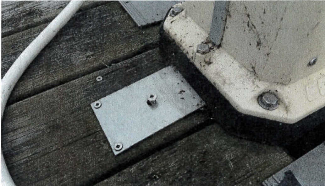
Photograph 141: West Main – Dock H. Pole at Slip 37 Connection Bolts Sticking Out
