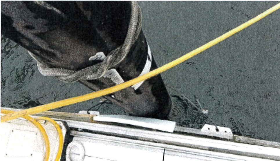
Photograph 124: West Main – Dock F. Pile 17. Steel Wire instead of Pile Guide. Welded Capping U Section and Bearing Pad Failed
