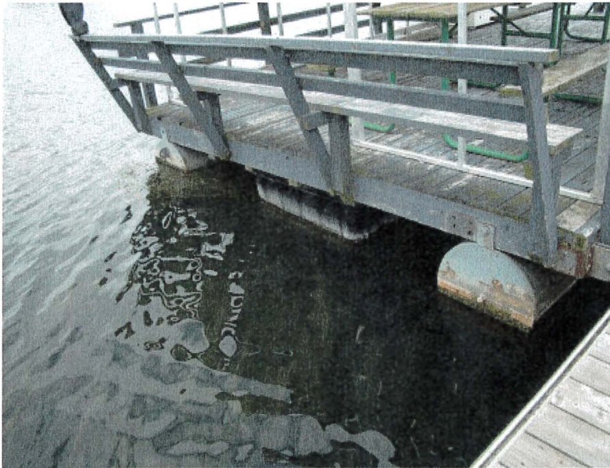
Photograph 39: East Main – Picnic Dock. Minor Superficial Corrosion on Steel Tubular Floats and Bolts
