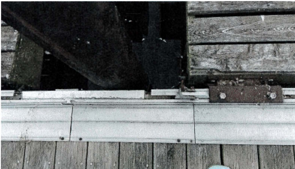
Photograph 160: West Main – Dock J. Launching Ramps. Bolted Connections Corroded
