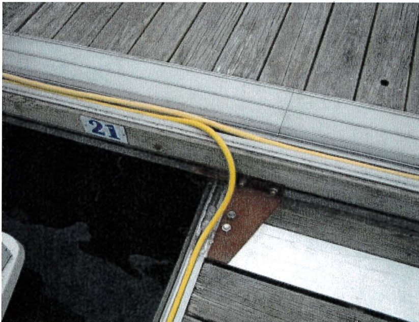
Photograph 112: West Main –Dock D. Base Plates Corroded in Finger 21/22
