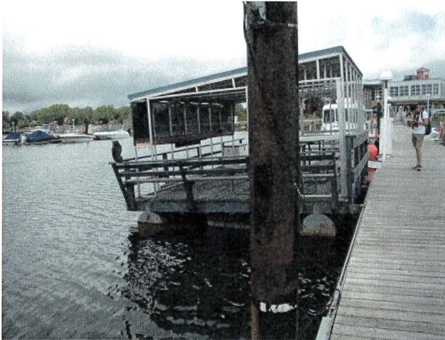
Photograph 37: East Main – Picnic Dock. Differential Elevation between Inner and Outer Sides
