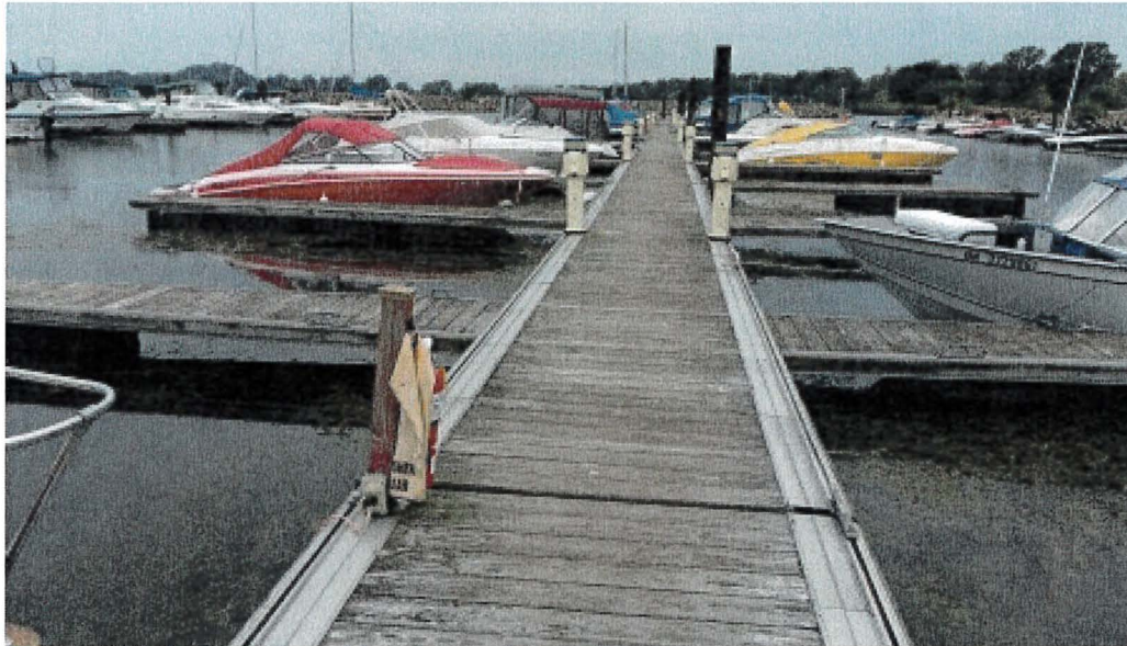
Photograph 149: West Main – Dock I. Loss of Pole at Slip 63
