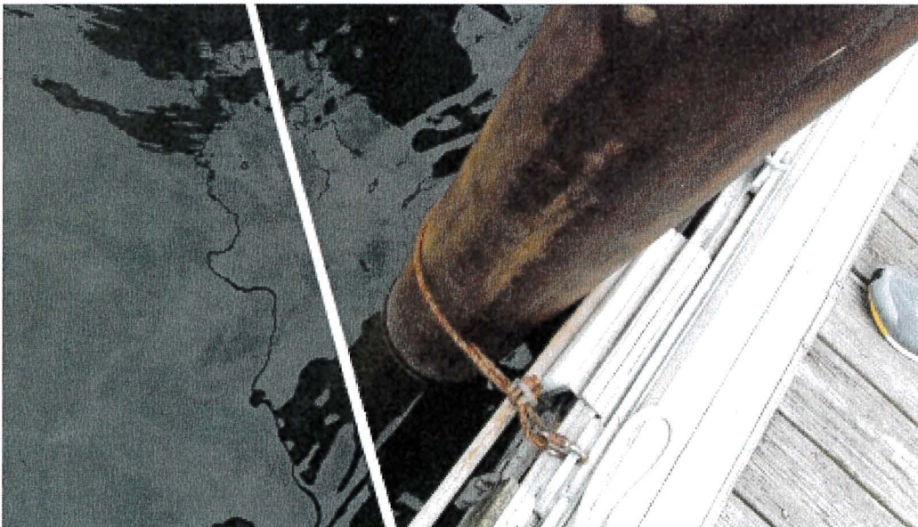
Photograph 118: West Main – Dock E. Pile 7. Steel Wire (Minor Superficial Corrosion) instead of Pile Guide
