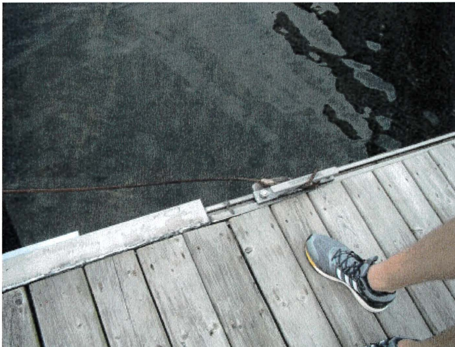
Photograph 40: East Main – Pile 4. Steel Wire instead of Pile Guide. Anchored to the Cleat Channel
