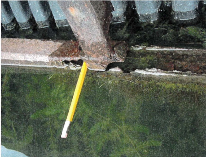
Photograph 53: East Main – Dock 4. Moderate to Heavy Corrosion of Steel Frame for Tubular Plastic Floats
