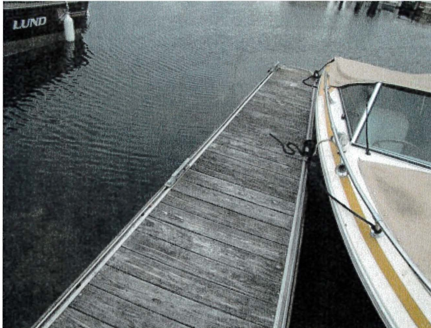
Photograph 87: West Main – Dock A. Deck Timber Minor Splintering by Slip 11
