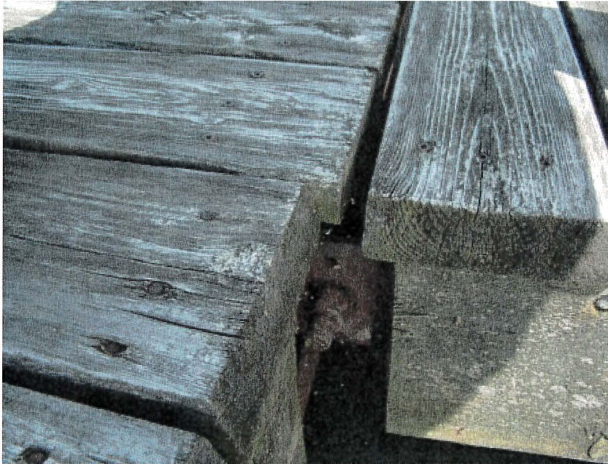
Photograph 51: East Main – Dock 3. Moderate Corrosion in most Bolted Connections between Floats
