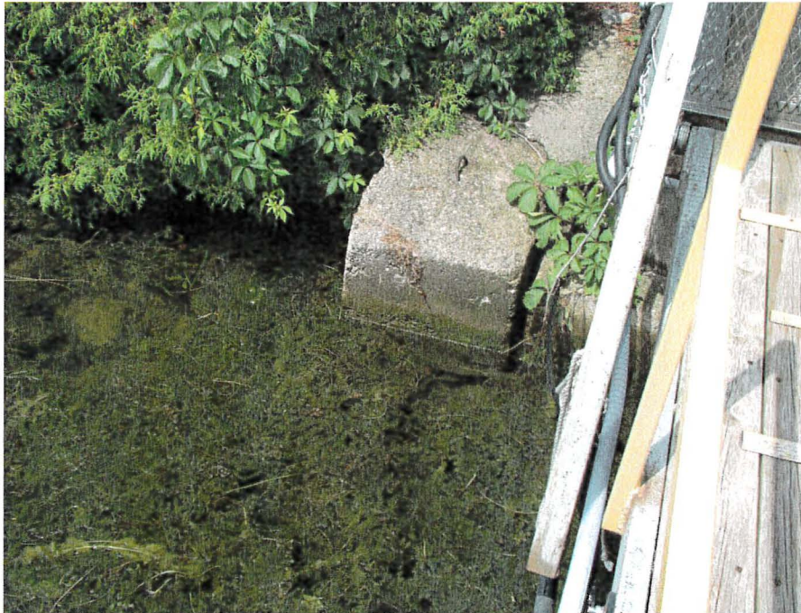
Photograph 7: Dock 1 – Abutment. NW Corner. Minor Cracks on the Concrete Surface
