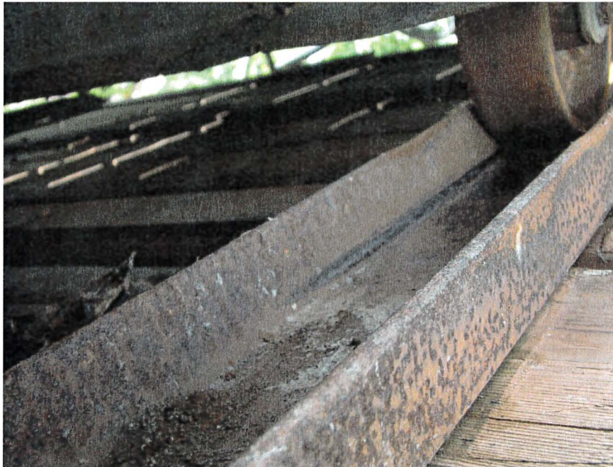
Photograph 9: Dock 1 – Access Gangway. Superficial Corrosion on Steel Beam and Roller Guides
