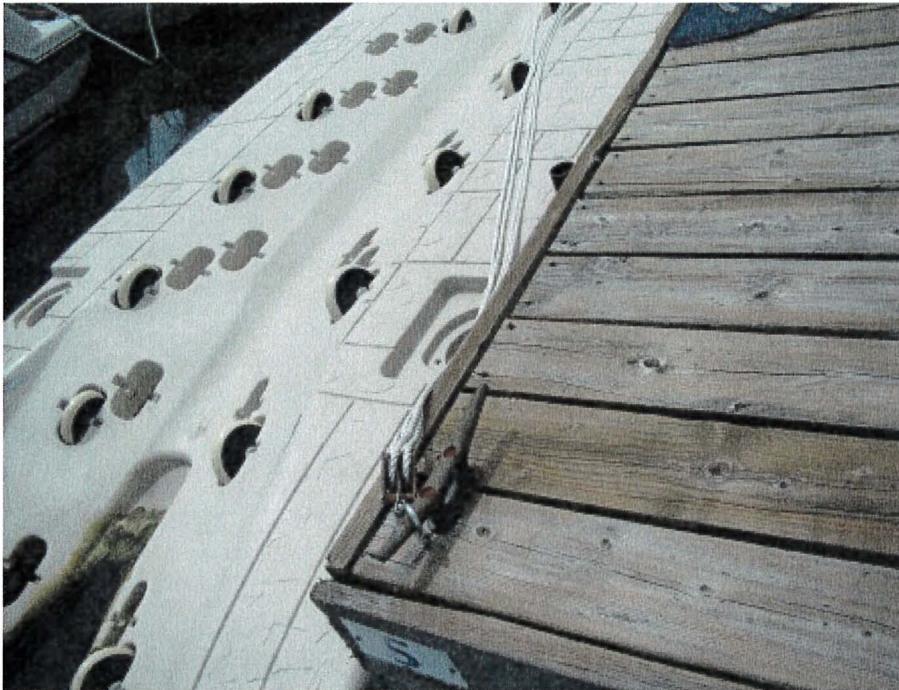
Photograph 11: Dock 1 – Finger 3/5. Bitts with Rusting in the Head of Anchorage Bolts
