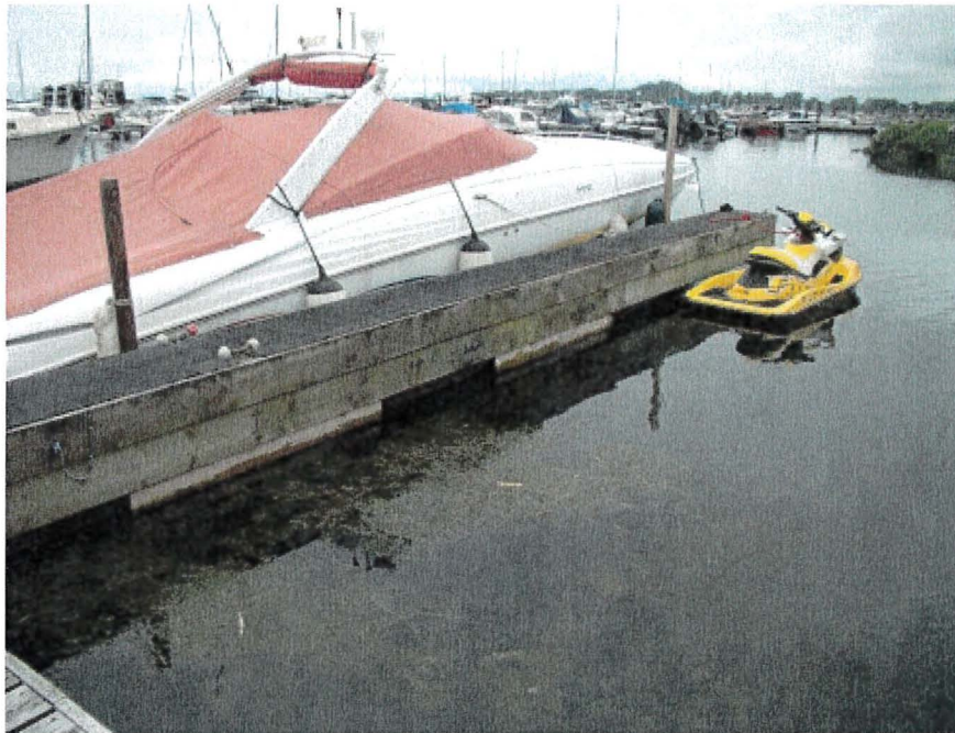
Photograph 27: Dock 2 – Finger 16/18. Moss Build-up. Surface Corrosion on Steel Cylinder Floats
