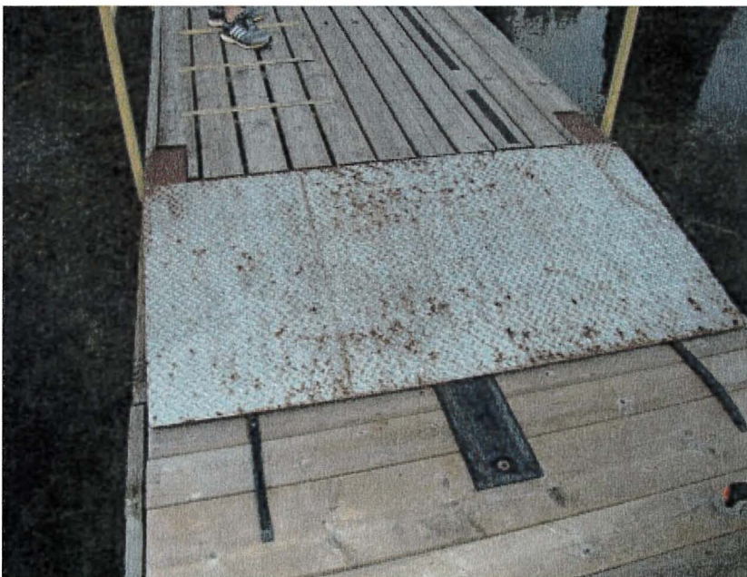
Photograph 20: Dock 2 – Access Gangway. Signs of Corrosion in the Base Plate
