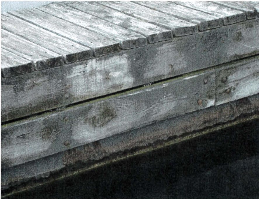
Photograph 62: East Main – Dock 6. Minor Surface Corrosion on Steel Floats
