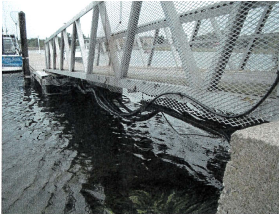
Photograph 69: West Main – Access Gate. Left Side View. Spalling on Concrete Abutment
