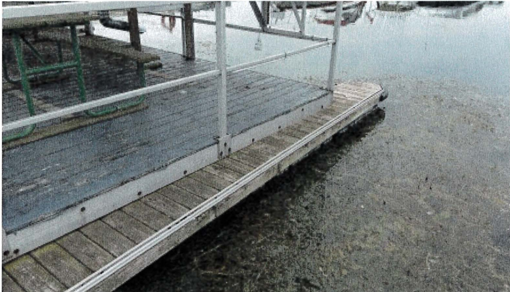
Photograph 153: West Main – Dock J. Fish Cleaning Dock. Minor Rotting of Deck Timbers.
