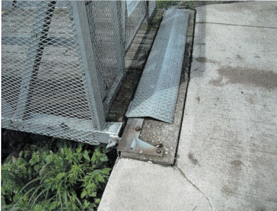
Photograph 31: East Main – Access Gate. Minor Signs of Corrosion in the Sheet of the Sill and Bolts
