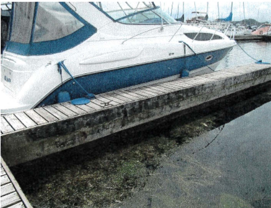
Photograph 12: Dock 1 – Finger 12/14. Moss Build-up. Surface Corrosion on Steel Cylinder Float
