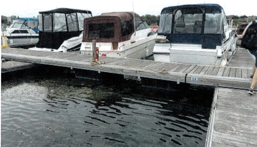
Photograph 140: West Main – Dock H. Pole at Slip 51 is Loose
