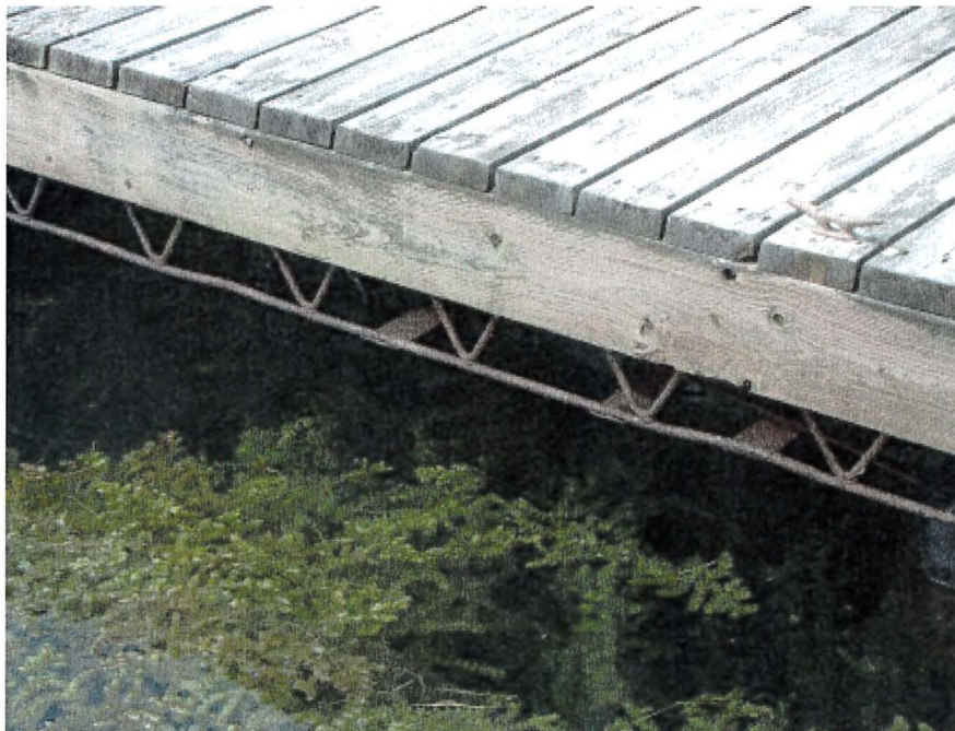
Photograph 49: East Main – Dock 3. Minor Deformation of Bottom chord of Steel Truss
