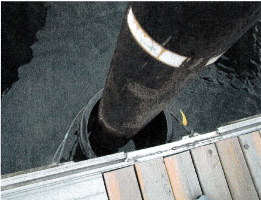
Photograph 94: West Main – Dock B. Pile 15. Steel Wire instead of Pile Guide.
