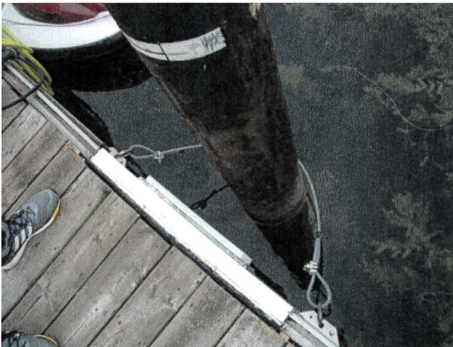
Photograph 74: West Main – Pile 2. Steel Wire instead of Pile Guide
