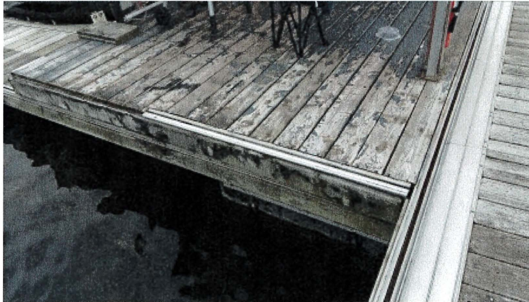
Photograph 137: West Main – Dock G. Minor Moss Build-up
