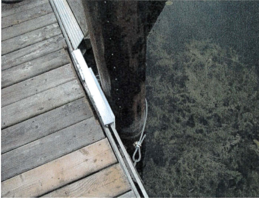
Photograph 75: West Main – Pile 3. Steel Wire instead of Pile Guide
