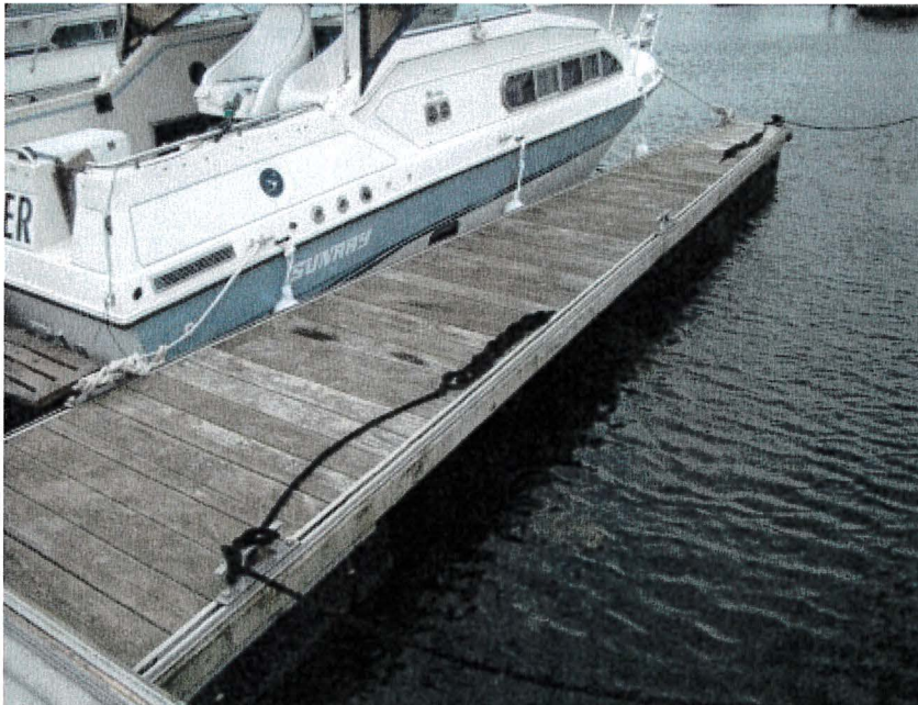
Photograph 114: West Main – Dock D. Moss Build-up on some Deck Timbers and Side Stringers
