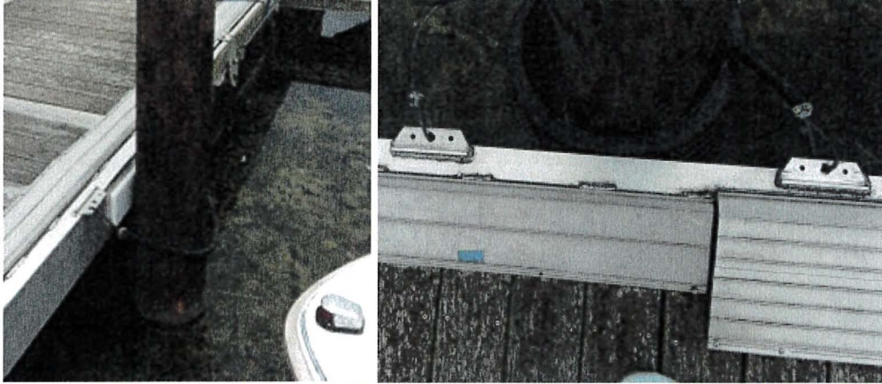
Photograph 157: West Main – Dock J. Steel Wire instead of Pile Guide in all Piles of the Dock. Wire anchored to the Welded Capping U Section
