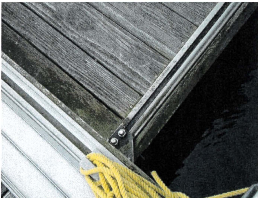
Photograph 92: West Main – Dock B. Moss Build-up on some Deck Timbers. Rotten Deck Timber (Slip 38)
