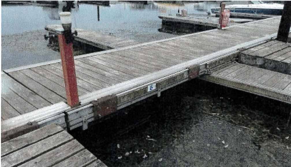
Photograph 161: West Main – Dock J. Corroded Plates in Slip 6
