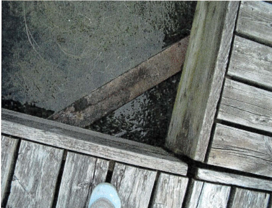
Photograph 25: Dock 2 – Finger 3/5. Surface Corrosion on Steel Beam underneath the Timber Deck
