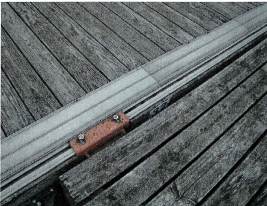
Photograph 96: West Main – Dock B. Corroded Bolt Washers at Slip 23
