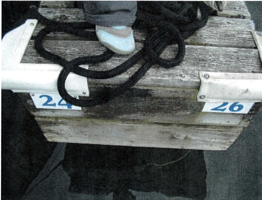
Photograph 29: Dock 2 – Finger 24/26. Edge of the deck. Rotten Timber
