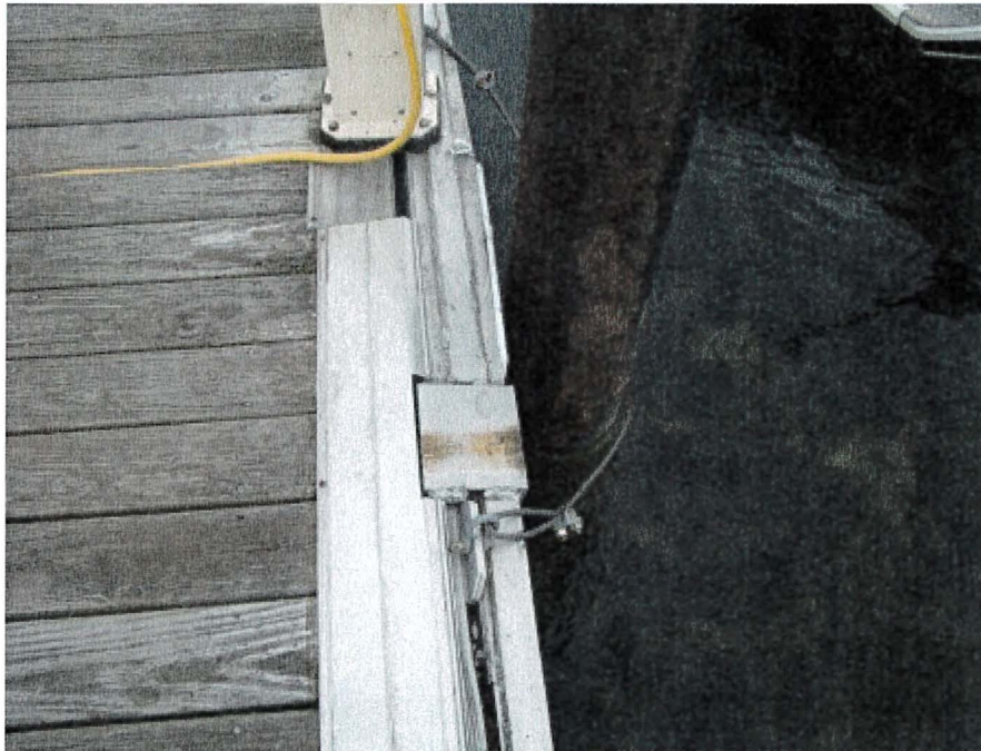
Photograph 99: West Main – Dock C. Pile 5. Steel Wire instead of Pile Guide
