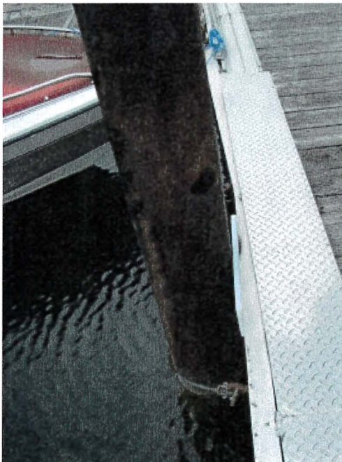
Photograph 84: West Main – Dock A. Pile 15. Steel Wire instead of Pile Guide. Welded Capping U Section Failed
