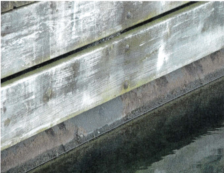
Photograph 60: East Main – Dock 5. Minor Surface Corrosion on Steel Floats
