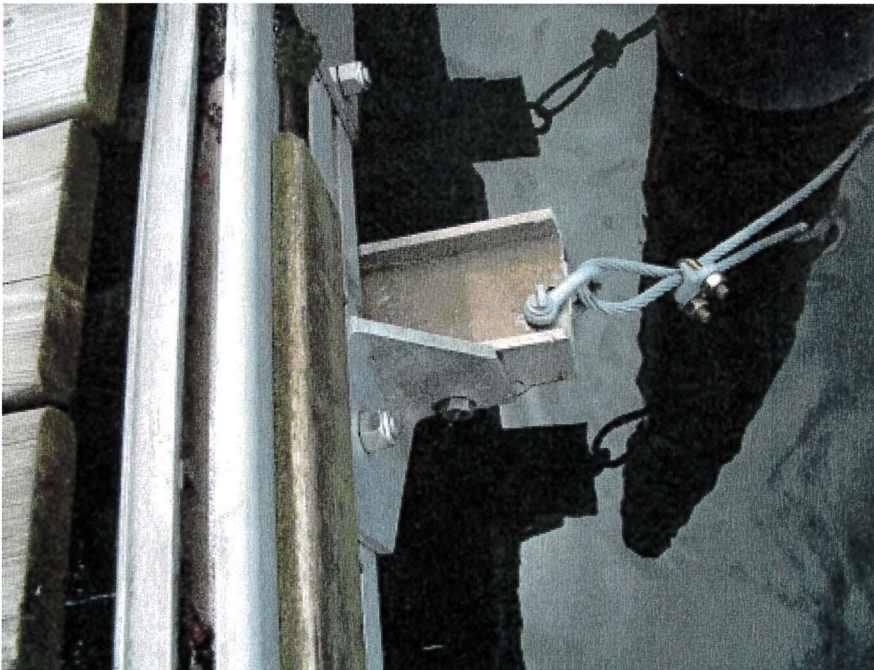
Photograph 36: East Main – Pile 1. Steel Wire instead of Pile Guide. Moss Build-up
