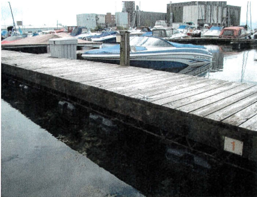
Photograph 47: East Main – Dock 3. Heavy Moss Build-up in Timber Supporting the Steel Truss
