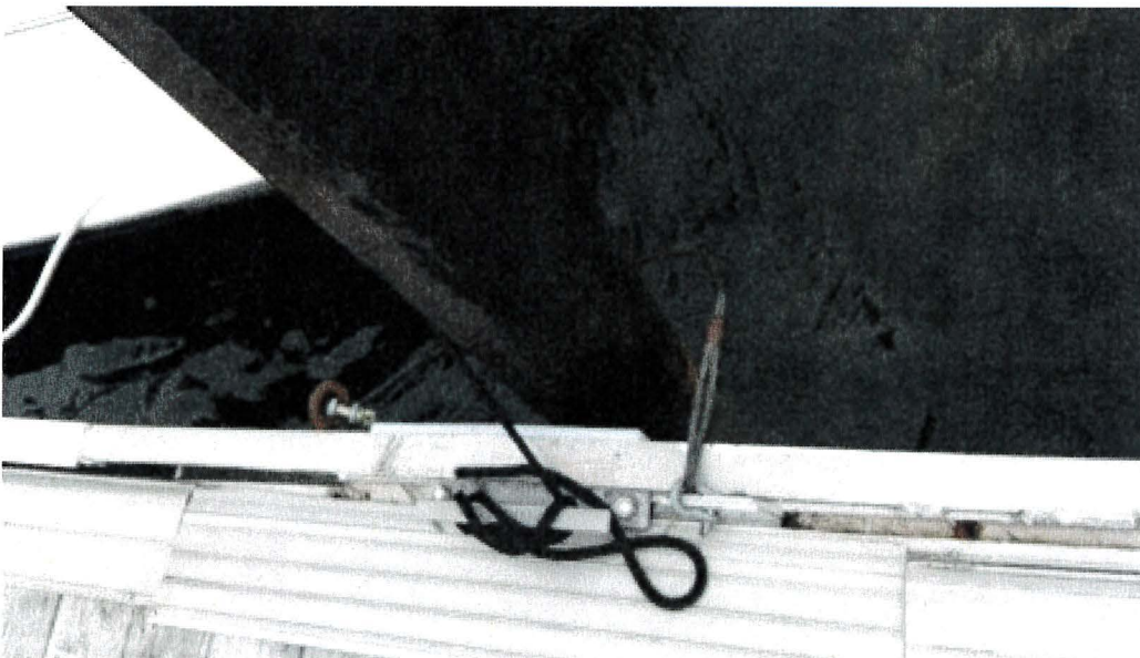
Photograph 122: West Main – Dock F. Pile 11. Steel Wire instead of Pile Guide. Welded Capping U Section and Bearing Pad Failed
