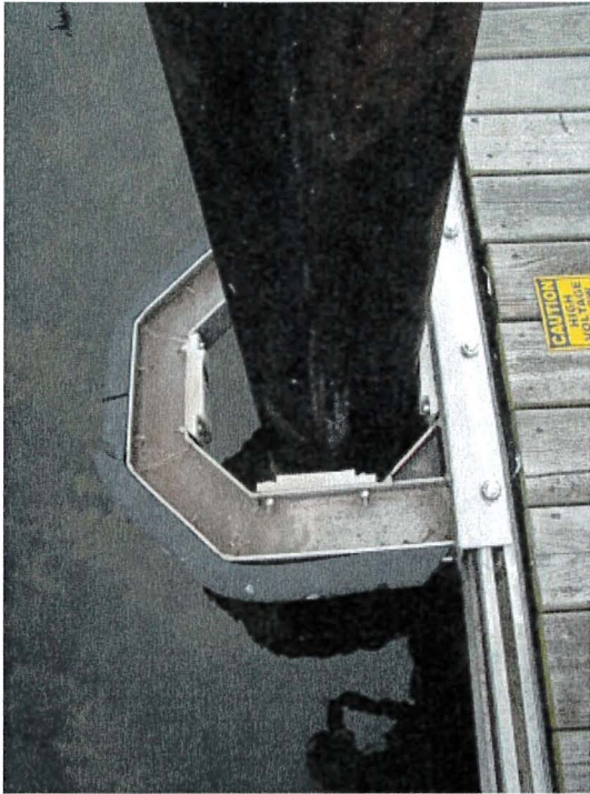
Photograph 77: West Main – Pile B-C. Rubber Fender Damaged and Inner Pads with Moderate Wear
