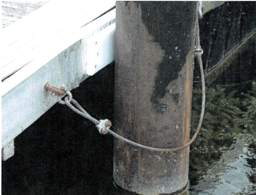
Photograph 83: West Main – Dock A. Pile 7. Steel Wire instead of Pile Guide. Welded Capping U Section Failed
