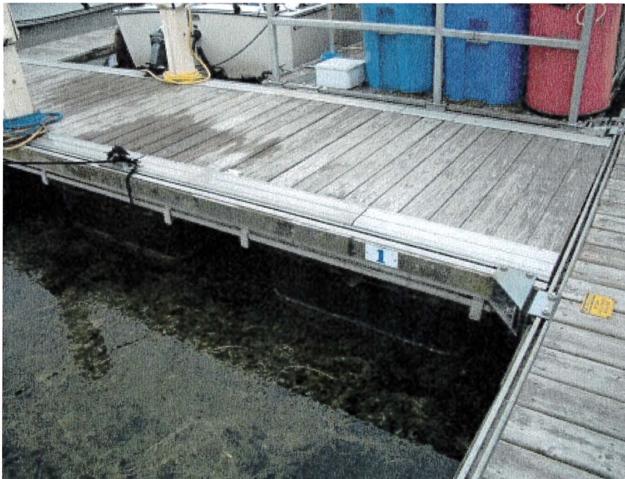
Photograph 98: West Main – Dock C. Moss Build-up on some Deck Timbers and Side Stringers
