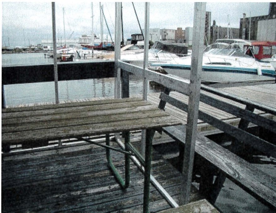
Photograph 38: East Main – Picnic Dock. Moderate Moss Build-up in Deck Timbers and Furniture
