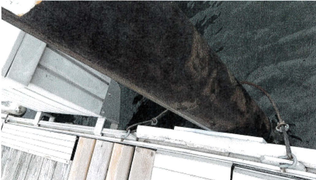
Photograph 117: West Main – Dock E. Pile 3. Steel Wire (Minor Superficial Corrosion) instead of Pile Guide
