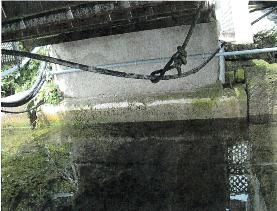
Photograph 5: Dock 1 – Abutment. Front View. Moss Build-up
