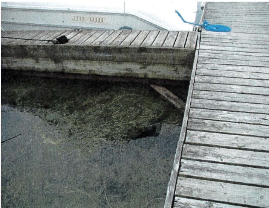
Photograph 24: Dock 2 – Timber Discoloration and Moss Build-up
