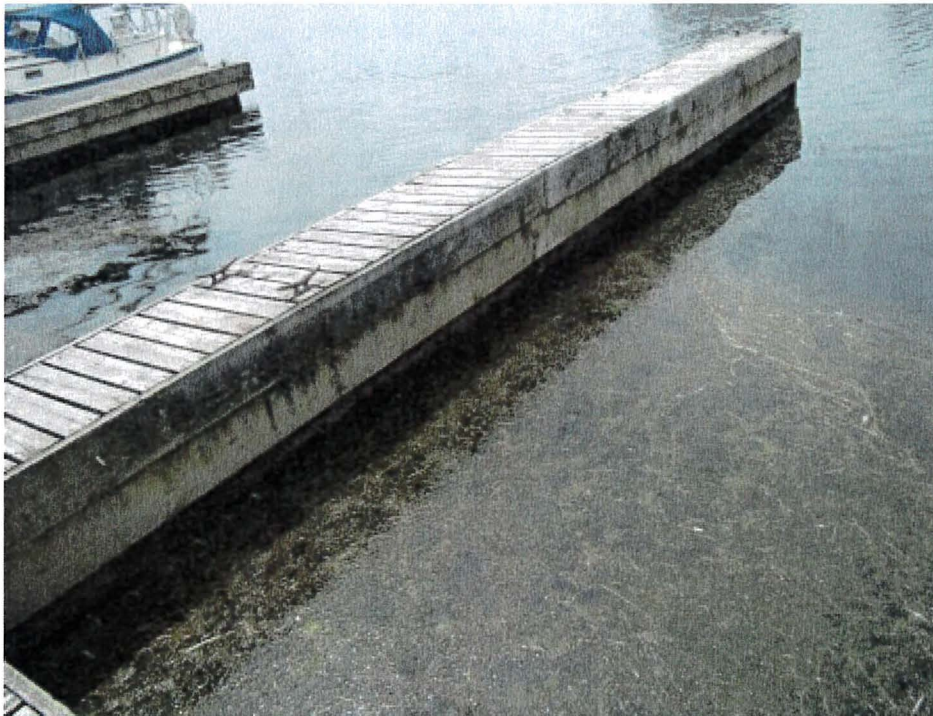
Photograph 16: Dock 1 – Finger 24/26. Surface Corrosion on Steel Cylinder Floats
