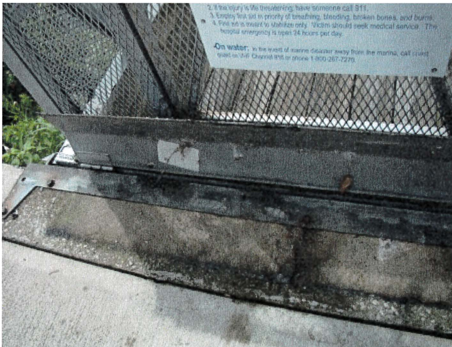
Photograph 32: East Main – Abutment. Desintegration on Top Face of the Connecting Slab
