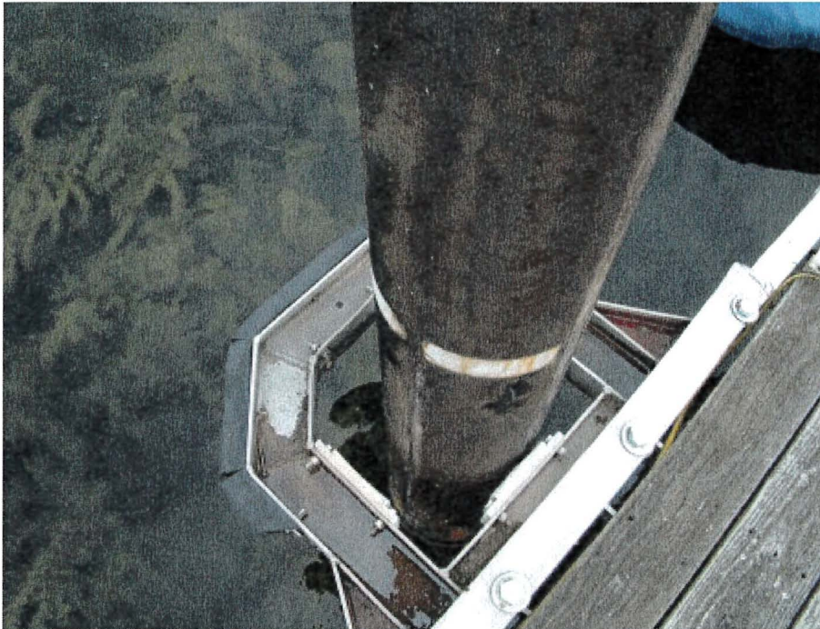
Photograph 95: West Main – Dock B. Pile-End. Inner Pads with Moderate Wear
