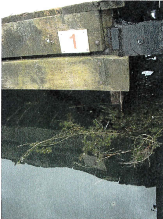
Photograph 59: East Main – Dock 5. Moss Build-up
