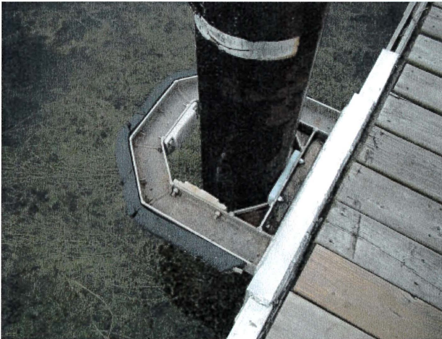
Photograph 76: West Main – Pile A-B. Rubber Fender Damaged
