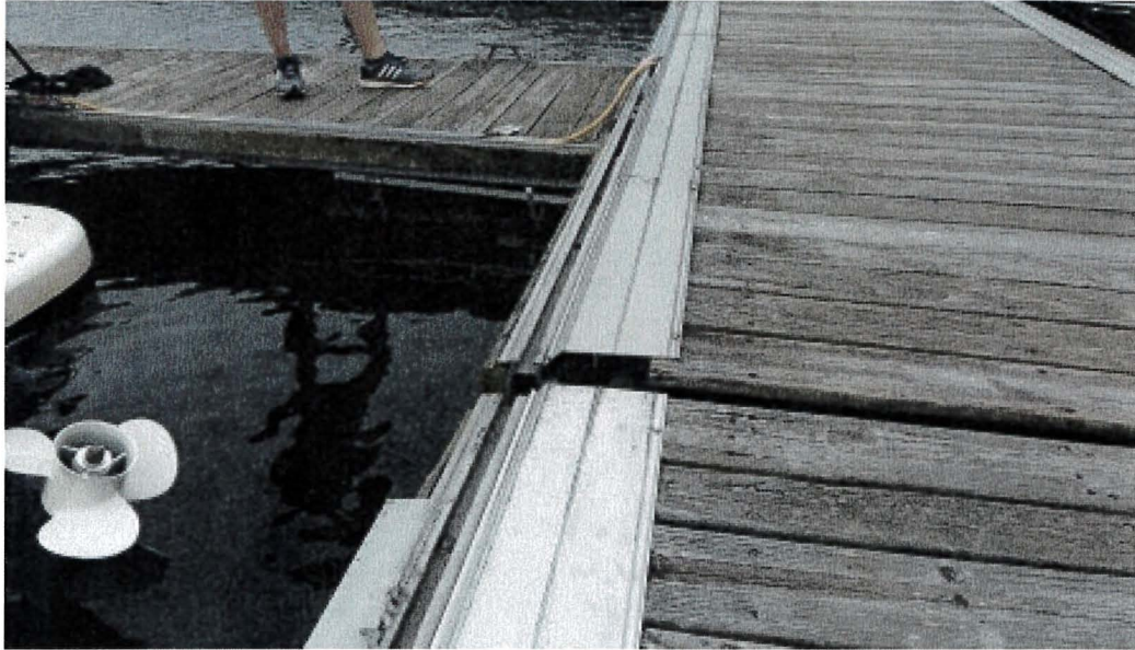
Photograph 135: West Main – Dock G. Differential Settlement between Slips 3 and 4
