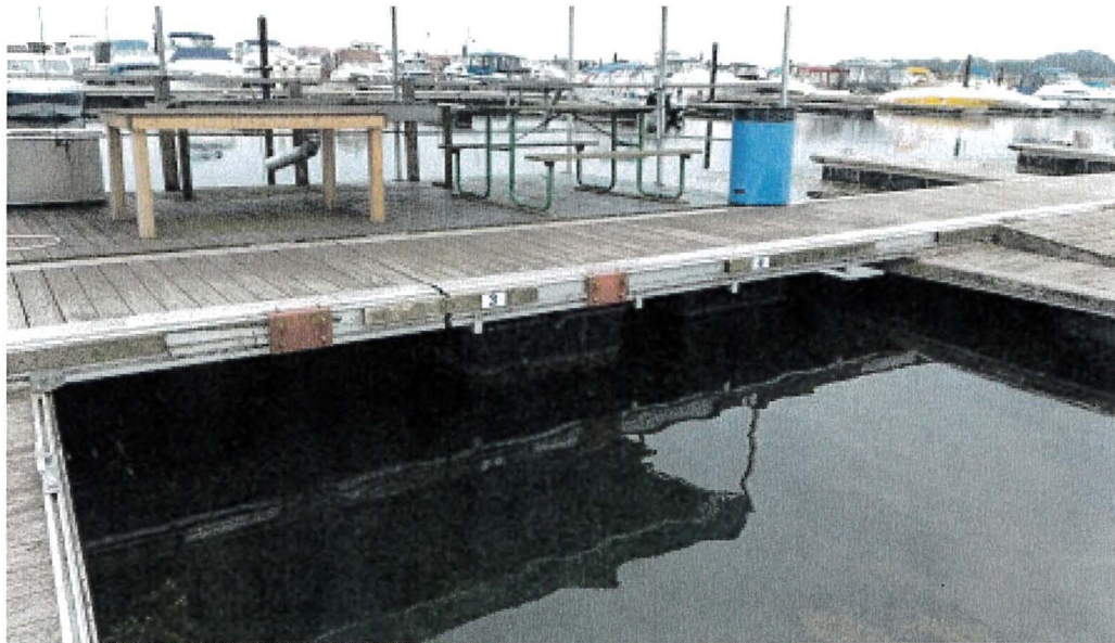
Photograph 151: West Main – Dock J. Fish Cleaning Dock. Differential Settlement between N and S
