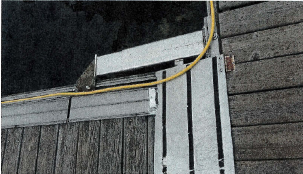
Photograph 145: West Main – Dock I. Very Steep Transition Plate. Minor Corrosion at Bolted Plates
