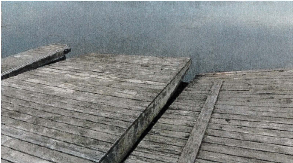
Photograph 159: West Main – Dock J. Launching Ramps. Loss of Flotation generally on West. Slips 5, 7 and 9
