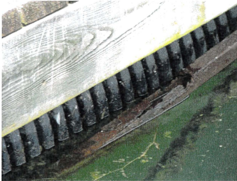
Photograph 57: East Main – Dock 4. Moderate to Heavy Corrosion of Steel Frame for Tubular Plastic Floats (5)
