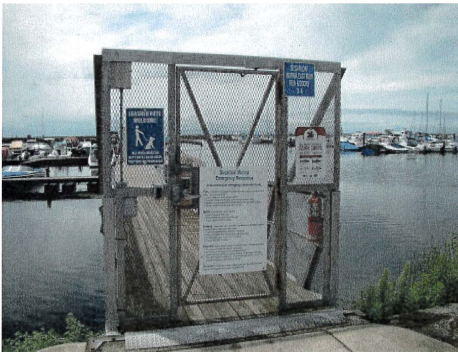
Photograph 66: West Main – Access Gate. Front View. Minor Corrosion on Hinges and Truss
