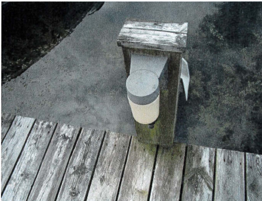
Photograph 50: East Main – Dock 3. Moderate Moss Build-up
