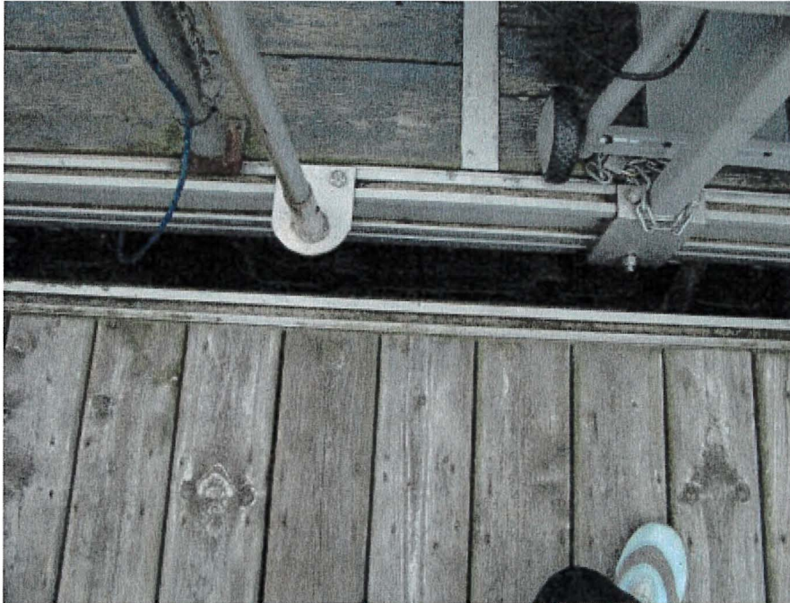
Photograph 103: West Main – Dock C. Picnic Dock. General Moss Build-up
