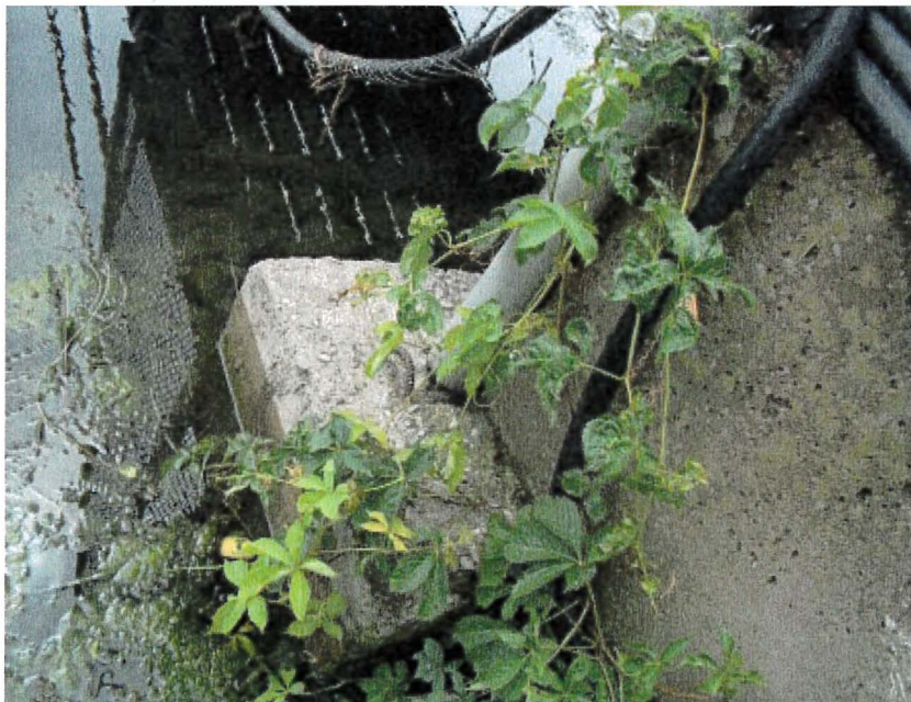
Photograph 18: Dock 2 – Abutment. Moderate Spalling
