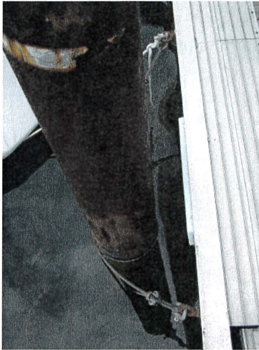
Photograph 109: West Main – Dock D. Pile 11. Steel Wire instead of Pile Guide
