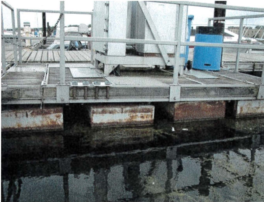
Photograph 89: West Main – Dock B. Minor Corrosion on Electrical Panel Floats
