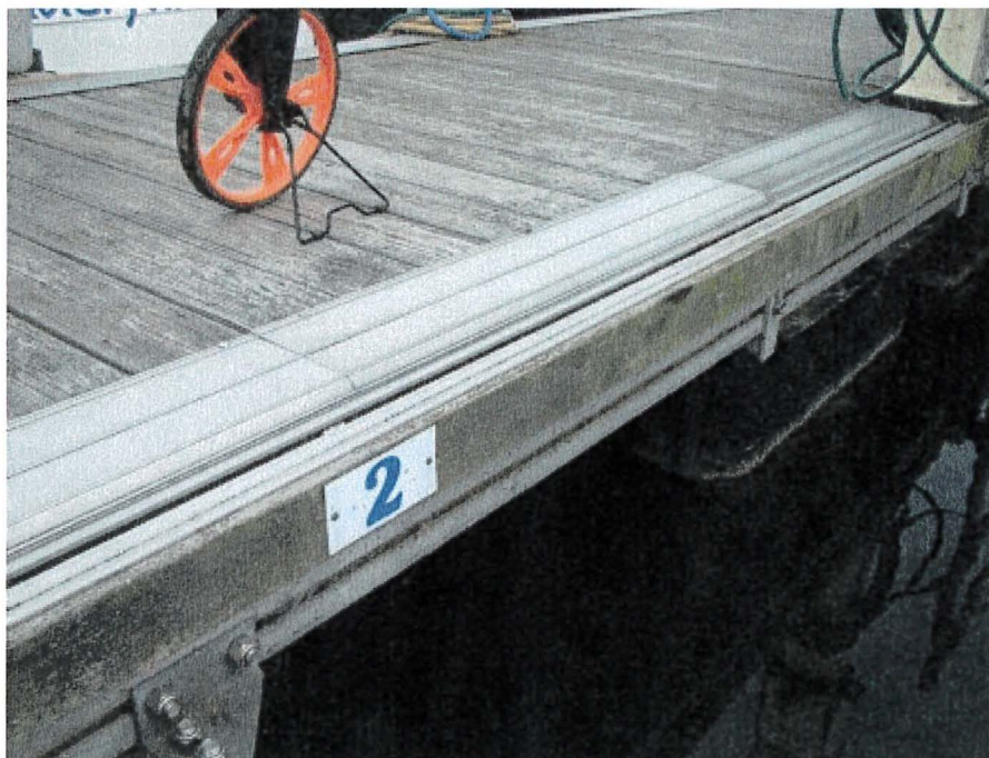
Photograph 91: West Main – Dock B. Moss Build-up on some Side Stringers
