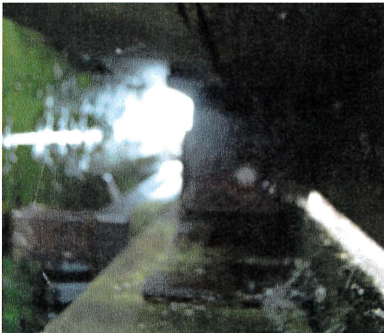
Photograph 58: East Main – Dock 4. Moderate Corrosion in Most Bolted Connections between Floats
