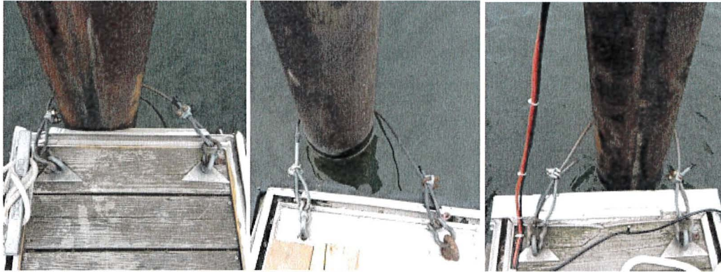
Photograph 119: West Main – Dock E. Piles of Fingers 10/11, 14/15, 16/17 without Pile Guide. Steel Wire anchored to the Deck Timber. Buckled Plate
