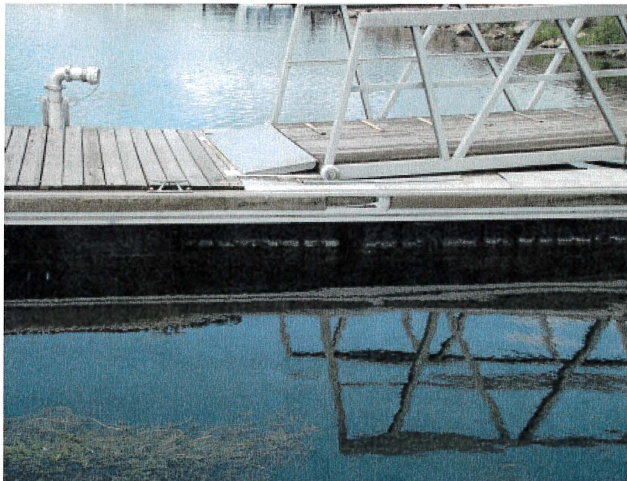
Photograph 34: East Main – Access Gangway. Loss of some Stringers
