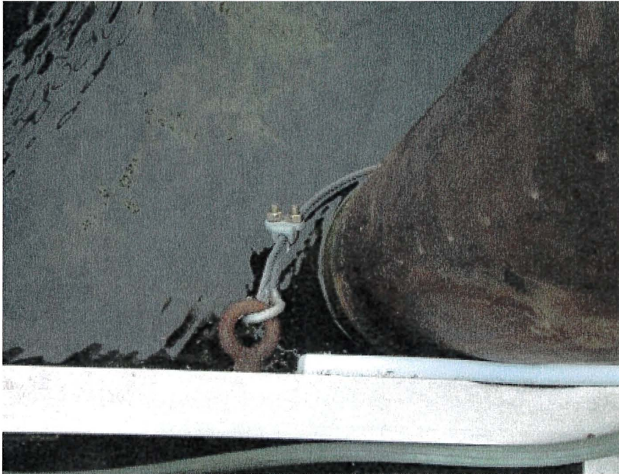
Photograph 93: West Main – Dock B. Pile 9. Steel Wire instead of Pile Guide.
