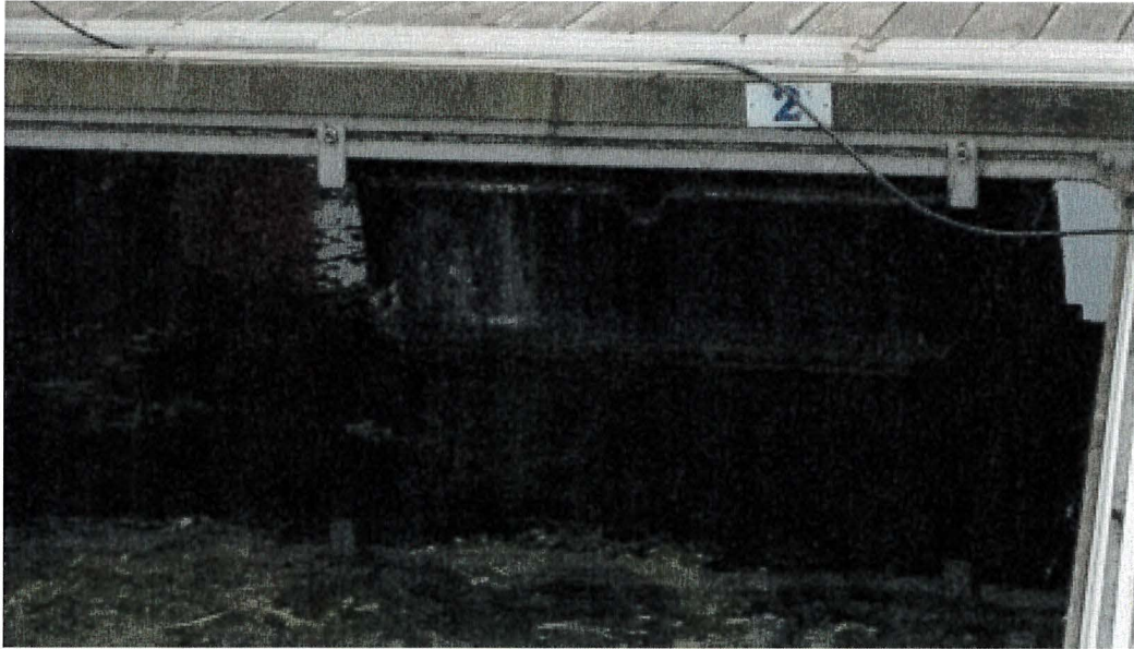
Photograph 147: West Main – Dock I. Minor Moss Build-up on Deck Timbers and Stringers
