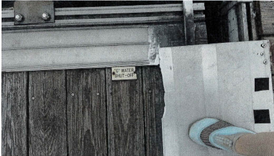
Photograph 133: West Main – Dock F. Loss of the East Side Panel at the End of Finger 30/31
