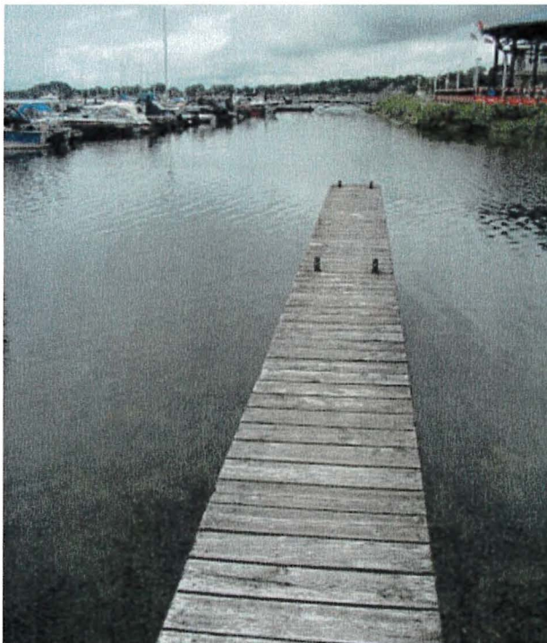
Photograph 28: Dock 2 –Finger 20/22. Timber Discoloration
