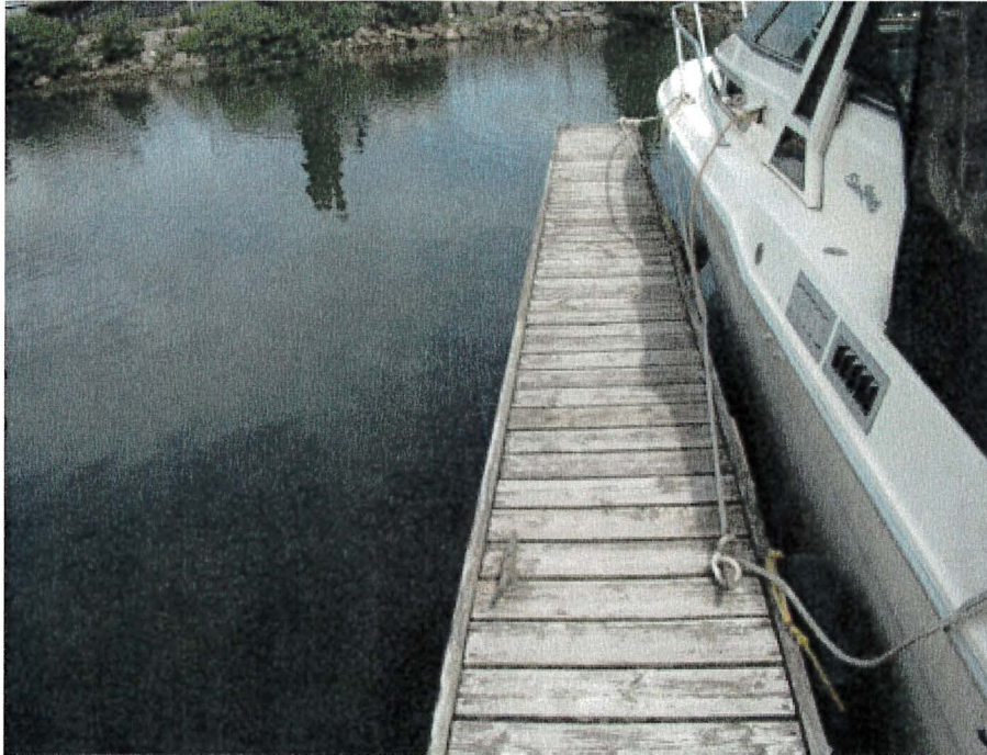
Photograph 13: Dock 1 – Finger 15/17. Timber discoloration
