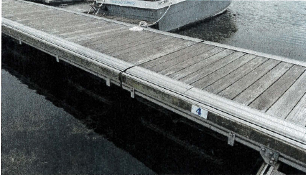
Photograph 139: West Main – Dock H. Moss Build-up
