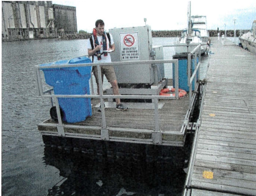
Photograph 43: East Main – Electrical Panel Float. Differential Elevation between Inner and Outer Side
