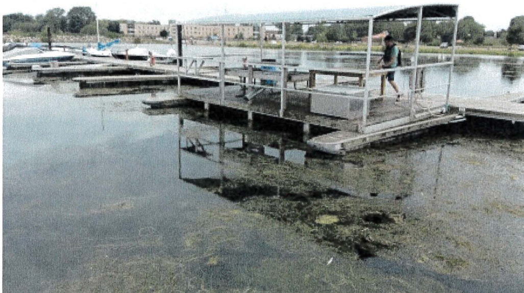
Photograph 152: West Main – Dock J. Fish Cleaning Dock. Supported by Fingers with Little Freeboard. Fender Hanging Loose on East Finger
