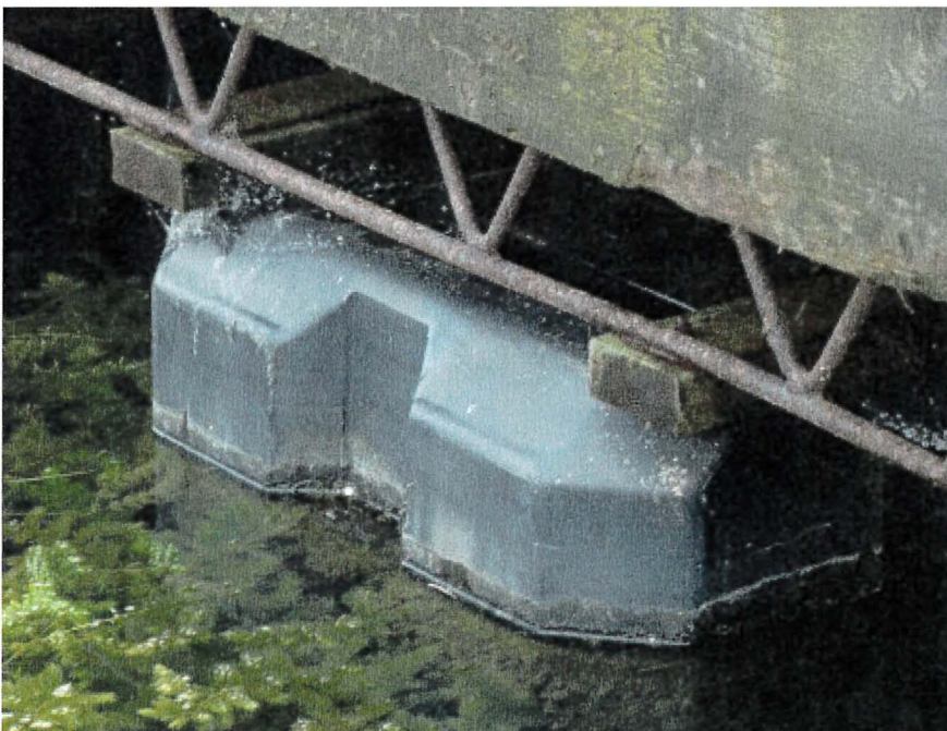
Photograph 48: East Main – Dock 3. General Corrosion of Steel Truss Supporting the Timber Deck
