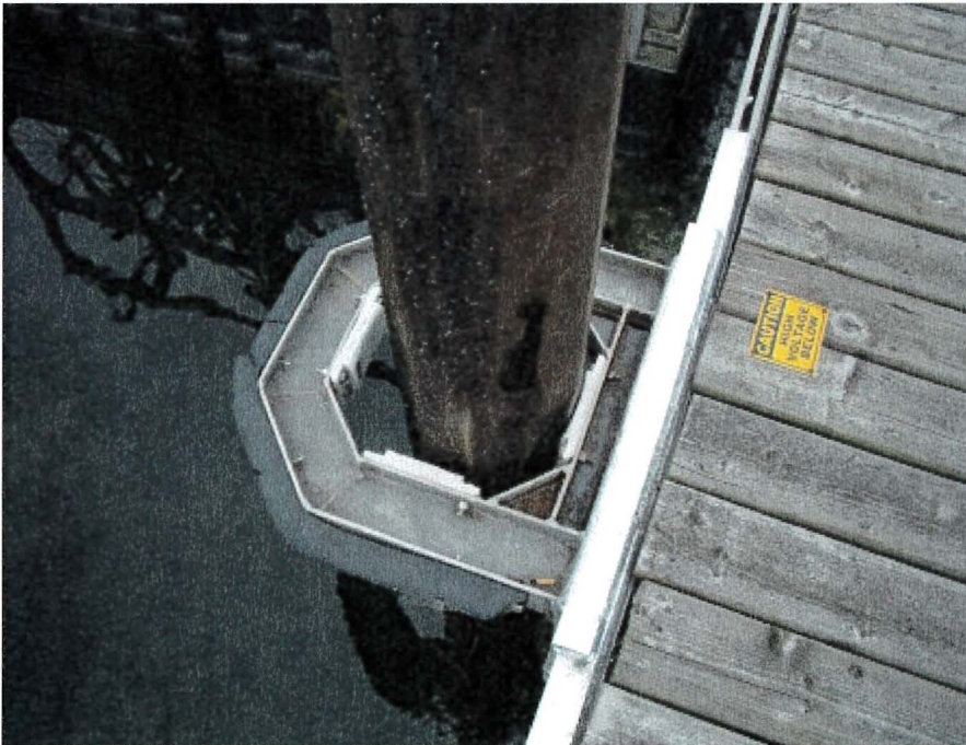
Photograph 78: West Main – Pile C-D. Rubber Fender Damaged and Inner Pads with Moderate Wear
